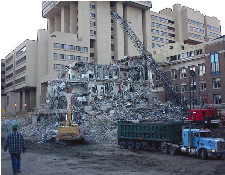
This demolition project near 10 health-care buildings on the University of Minnesota campus was preceded by an extensive ICRA.
